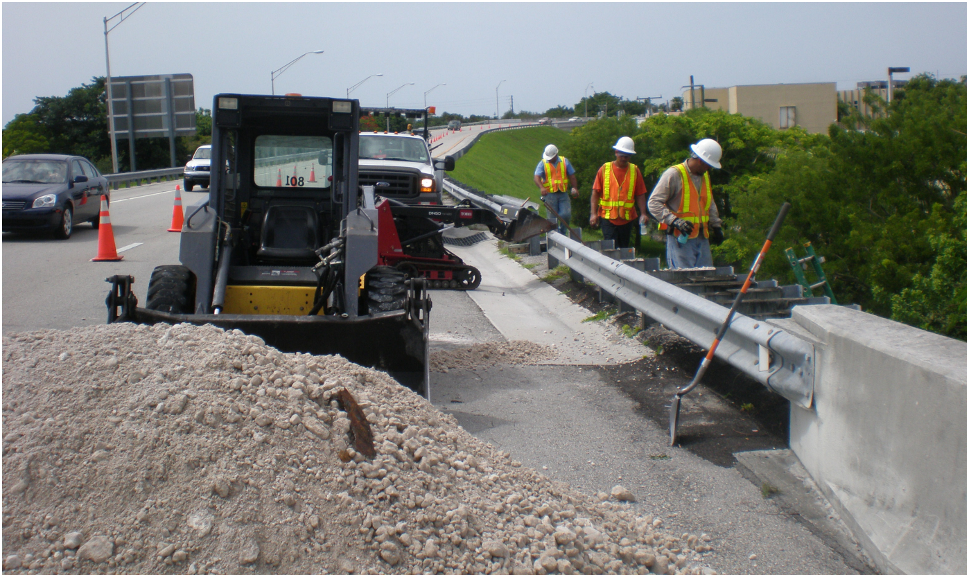
FIGURE 20: EXAMPLE OF CREW PERFORMING SLOPE REPAIR ALONGSIDE THE APPROACH TO A BRIDGE
