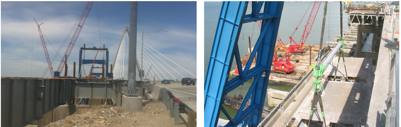
FIGURE 34: DEMOLITION OF THE EXISTING BRIDGE IN CLOSE PROXIMITY TO THE REPLACEMENT BRIDGE ON THE CHRISTOPHER S. BOND BRIDGE PROJECT (LEFT). GALVESTON DEMOLITION OF EXISTING BRIDGE (RIGHT)
