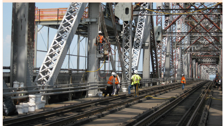
FIGURE 48: URBAN ENVIRONMENT - MID-POINT RETROFIT ACCESS FROM SPIDERS ON RAIL SIDE ON ROAD SIDE HUEY P. LONG PROJECT
