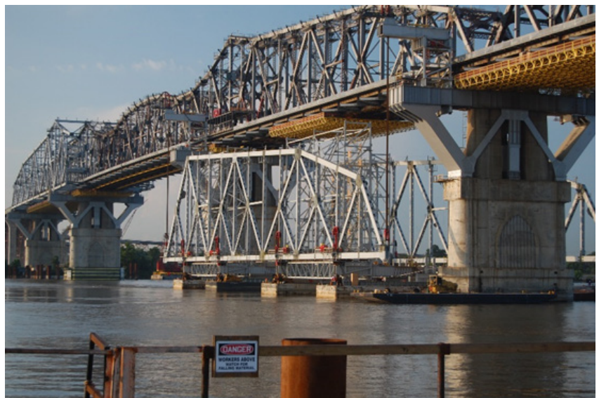
FIGURE 36: TRAYLOR AND MASSMAN WORKED CLOSELY WITH THE U.S. COAST GUARD AND OTHER MARITIME STAKEHOLDERS DURING THE INNOVATIVE LIFT OF THE MAIN SPAN TRUSS STRUCTURES ON THE HUEY P. LONG BRIDGE
