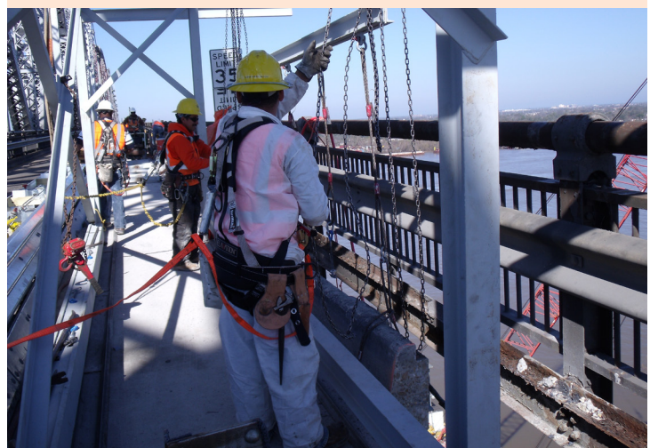
FIGURE 50: PROPER SAFETY PROCEDURES AT THE HUEY P. LONG PROJECT WHILE REMOVING CURB SECTION WITH DEMO CART
