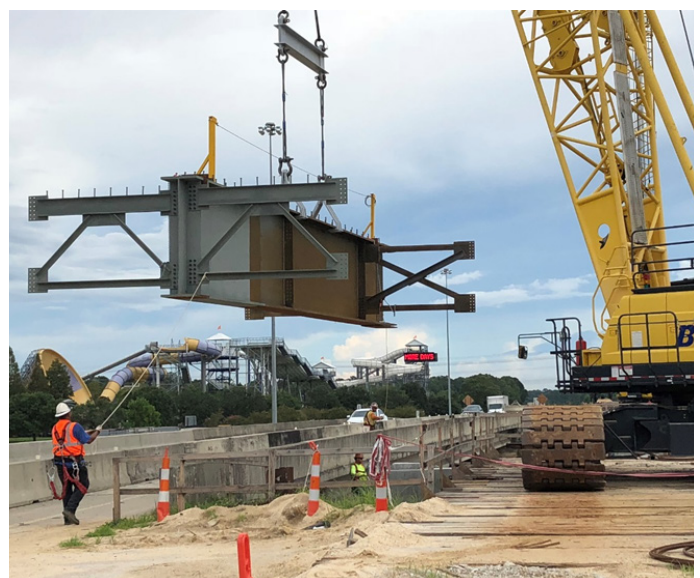
I-10 DESIGN BUILD LA 73 TO HIGHLAND, EAST BATON ROUGE TO ASCENSION, LA
