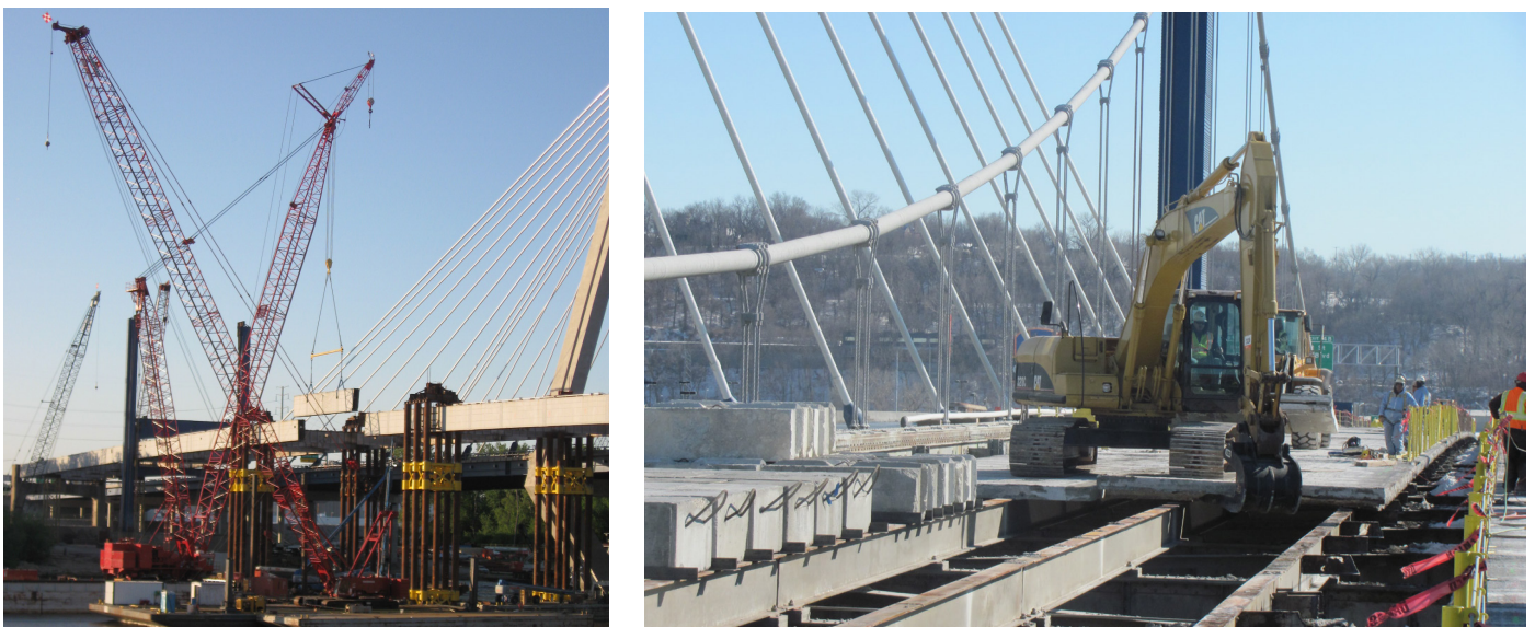
FIGURE 35: REMOVAL OF STRUCTURAL STEEL AND CONCRETE DECK OVER A NAVIGABLE WATERWAY DURING THE DEMOLITION PHASE OF THE CHRISTOPHER S. BOND BRIDGE PROJECT
